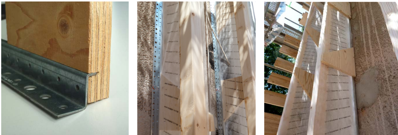
Image 4: Detailed view of the console and the metal rail (left), mounting of the substructure at the existing wall (centre + right)
