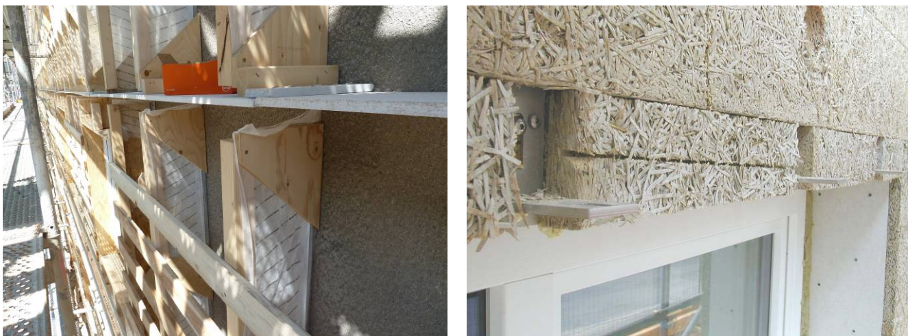
Image 5: Detailed view of the separation between the floors with a fire protection panel, still without the mineral insulation plate (left), brackets for mounting the shading on the insulation structure, which is possible easily (right)
